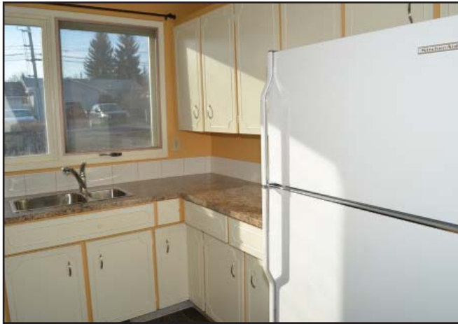
New counter-tops in the kitchen, new double sink and hardware on the cabinetry.
